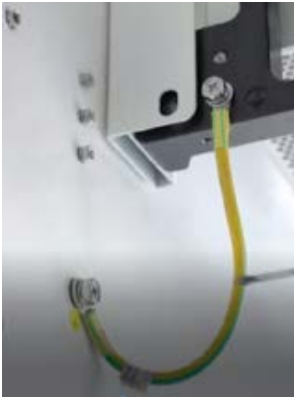
Figure 7-6 Ground connection with cabinet enclosure
