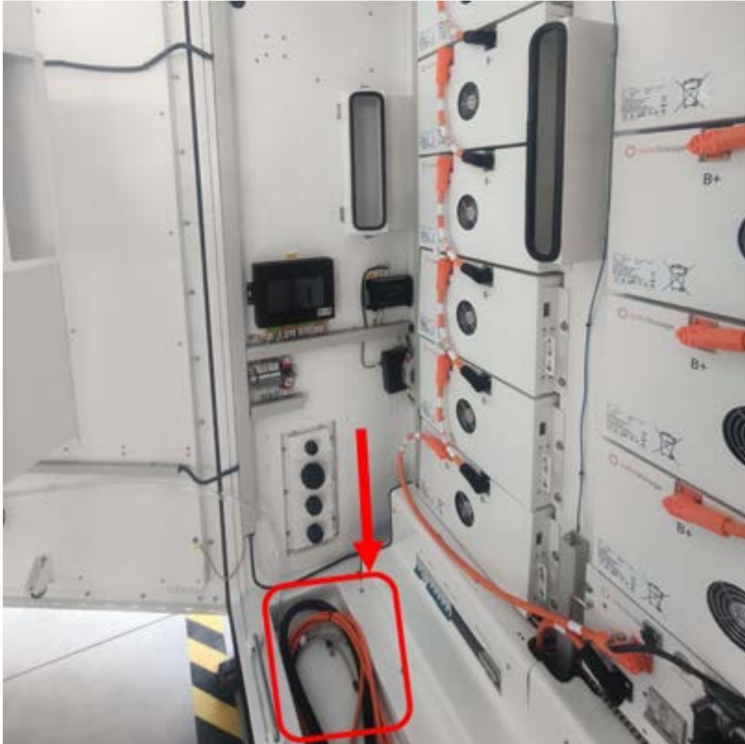
Figure 6- 1 Pre-installed cables inside cabinet
